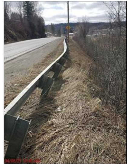
Figure 2: Compromised guardrail high above a steep slope along the road.
